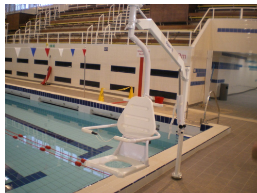
One of the new hoists
